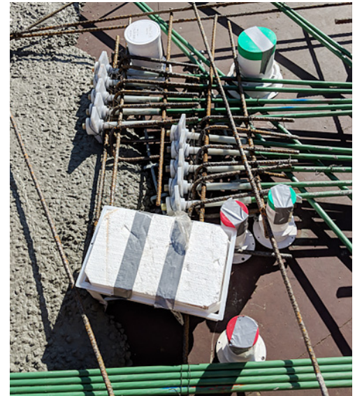
Fig. 2.750: PT anchors adjacent to Schedule 40 sleeves. (Image courtesy of Amsysco.)
