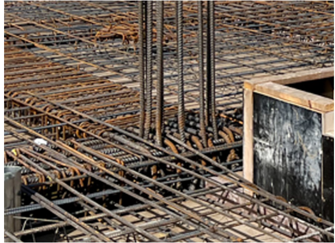
Fig. 2.7.20: Reinforcing bars at a beam-slab-column connection (photo courtesy of Ceko Concrete Construction.) Note that ACI 318 Section 24.3.4 requires tension reinforcement in beam and girder flanges (top bars at column intersections) to be distributed within the lesser of the effective flange width b_f or a width equal to 10% of the clear span l_n of the flexural member (refer to Fig. 2.7.27).
