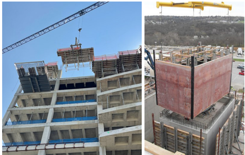
Fig. 2.6.8: Movement of panelized formwork systems requires crane time, capacity, reach and clear area below the load when beyond the building perimeter: (a) lifting a perimeter table panel to the next level; and (b) hoisting an interior core wall gang form. (Images courtesy of Ceco Concrete Construction.)
