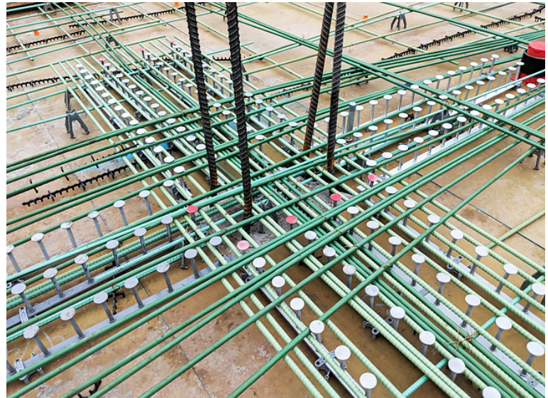
Fig. 2.748: Stud rails or double-headed studs can help designers avoid the need for drop panels. (Image courtesy of Amsysco.)
