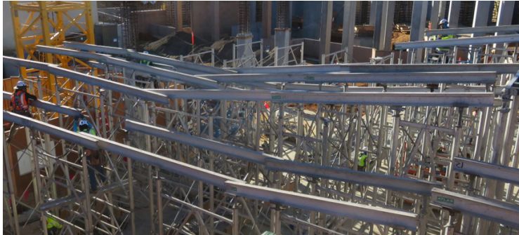
Fig. 2.6.28: Straight-soffit formwork elements are used to achieve a one-way slope transition with high shoring. While the formwork for such a transition is complex, it is more constructable than the formwork required to create a two-way slope or a warped slab. (Image courtesy of Hensel Phelps.)
