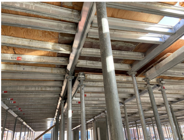
Fig. 2.6.33: Slab soffit offsets require interruption of the formwork framing, forcing the need for additional shores, labor, and time. (Image courtesy of Ceco Concrete Construction.)
