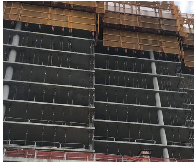
Fig. 2.6.45: A floor required to support mechanical equipment, a swimming pool, or to transfer loads to create a column-free space will have a high dead load, requiring a high quantity of reshores that will delay the work of interior trades (photo courtesy of Conco).
