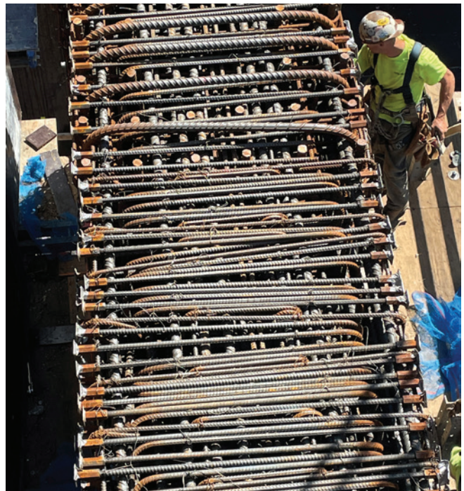
Fig. 2.7.1: The reinforcement in this member approached 800 lb/yd 3 and clearly presented a constructability challenge. (Image from “ Reinforcement Congestion in Cast-in-Place Concrete ,” Concrete International, December 2022 ( ascconline.org ),)
