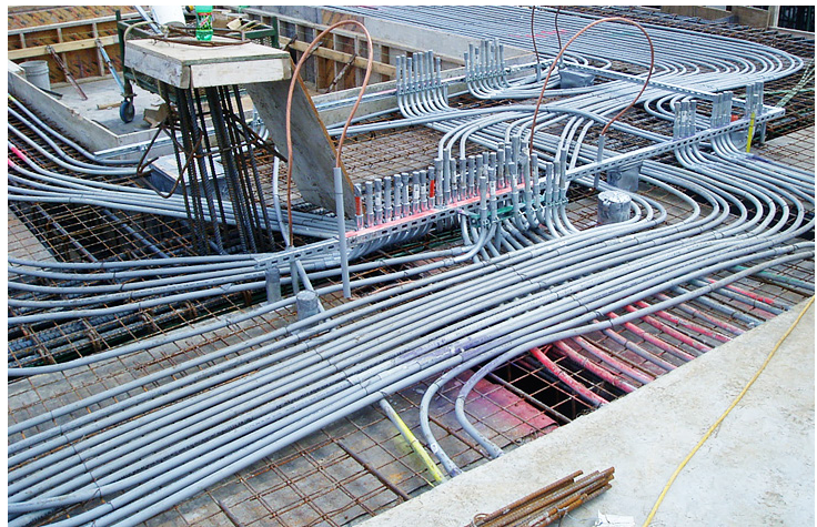
Fig. 2.7.41: This heavy concentration of electrical conduit conflicts with vertical reinforcement and will make it almost impossible for concrete to flow between the conduit and the forms below. (Image courtesy of Ceco Concrete Construction..)
