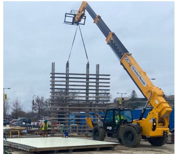
Fig. 2.6.5: Workers engage in the make-up of a large gang form. Larger panels require onsite labor, area, time and hoisting to support the make-up. Further, they are too large to assemble off site and truck to/from the site. A similar disassembly process is required upon completion of use. (Image courtesy of Ceco Concrete Construction.)
