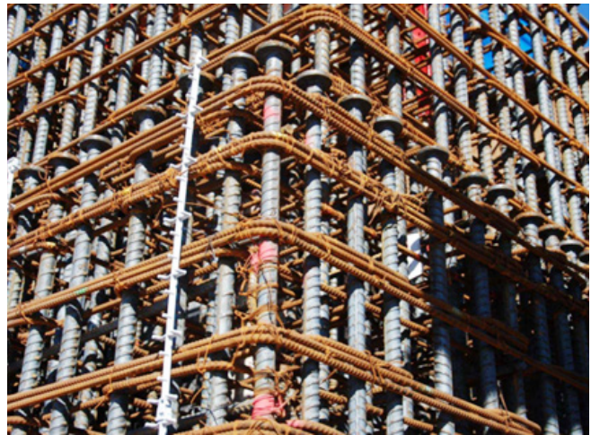
Fig. 2.7.3: An example of a shear wall reinforcing cage that has been detailed for constructability. (Image courtesy of Headed Reinforcement Corp.)
