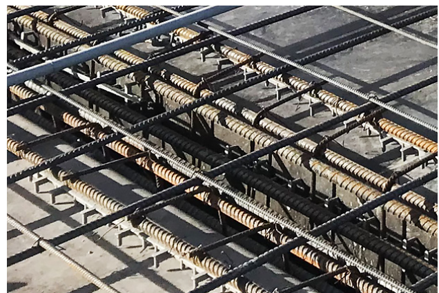
Fig. 2.7.22: Beam stirrups having out-turned hooks and open tops enable concrete placement and consolidation. Other constructable solutions include stirrups comprising baskets fabricated using welded-wire reinforcement. (Image courtesy of Ceko Concrete Construction.)
