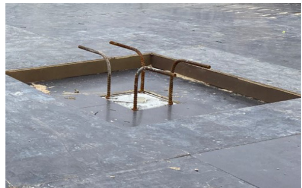
Fig. 2.6.34: A drop panel has been formed and is awaiting reinforcement installation. Better constructability is achieved using shear studs in lieu of a drop panel (refer to Section 2.7(h)). (Image courtesy of Ceco Concrete Construction.)
