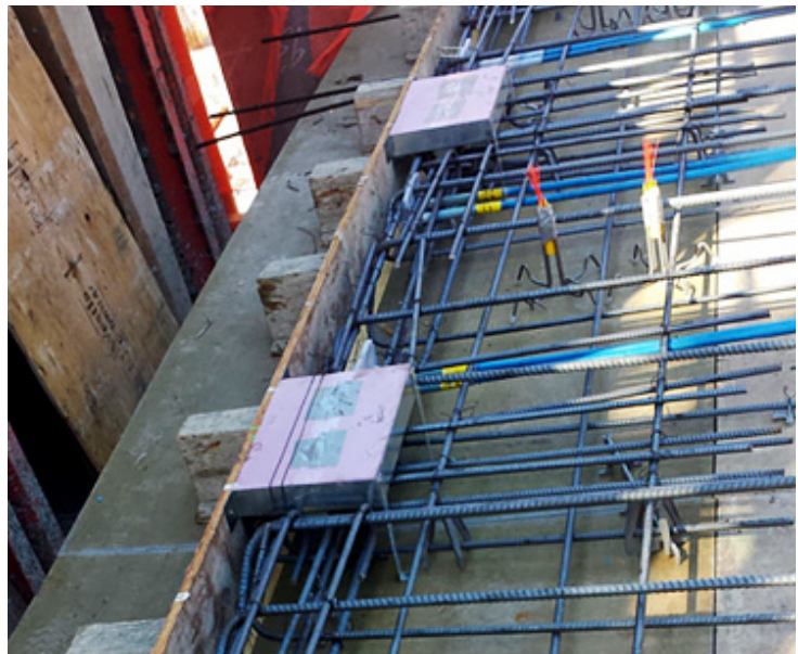
Fig. 2.7.42: Cladding connection systems are not all typical and should be considered for constructability in the reinforcing design as they may reduce clearance or displace reinforcement. (Image courtesy of CKC.)
