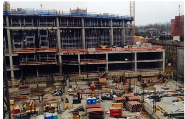
Fig. 2.6.15: A project with a tower structure isolated from a base structure. The separation followed a straight column line rather than the radius of the tower. (Image courtesy of Ceco Concrete Construction.)
