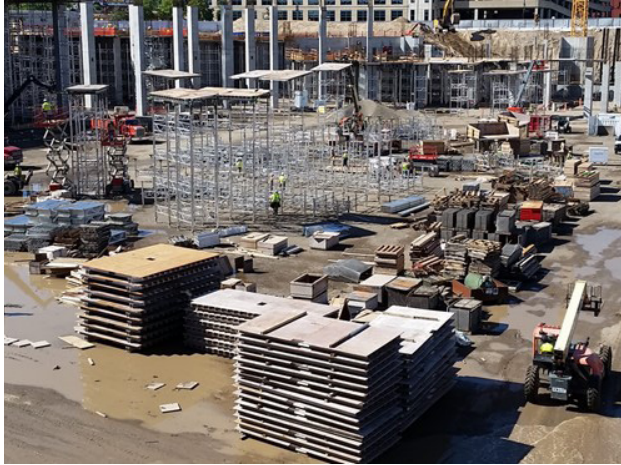
Fig. 2.6.13: A project “boneyard” of idle formwork. (Image courtesy of Ceco Concrete Construction.)
