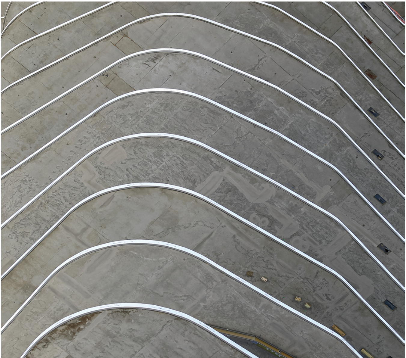
Multi-story high-rise undulated slab edge completed through constructable design practice. (Image courtesy of Ceco Concrete Construction.)
