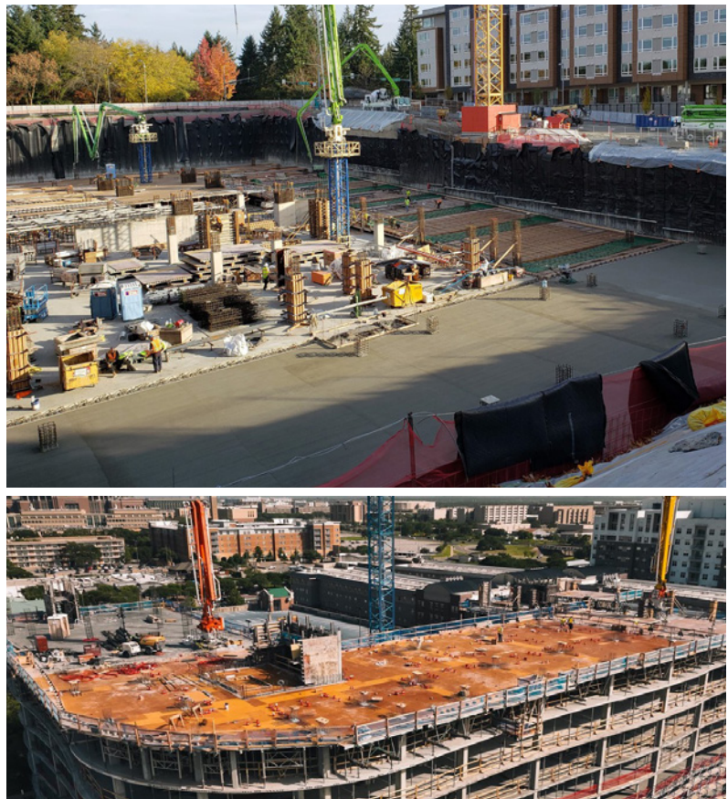
Fig. 2.6.6: Ideally, sufficient formwork should be available to place concrete in one section, place reinforcing in a second section, and complete curing and formwork removal in a third section. A three-pour concept, as shown in these examples, is desired by contractors to provide labor force and labor task continuity. Both benefits will increase productivity of the crew and individual craft personnel, maximizing their progression on the learning curve (refer to Fig. 2.4.4). (Images courtesy of Conco (top) and Ceco Concrete Construction (bottom).)
