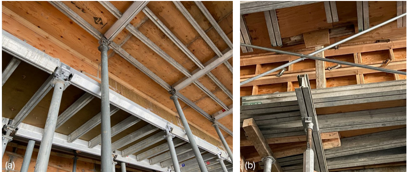
2.6.19: Photos of forms with beam sides connecting beam bottoms with slab soffits: (a) form depths of 20 in. or less allow form sides to carry concrete pressures with minimal members (photo courtesy of Ceco); and (b) form depths exceeding 20 in. necessitate studs, wales, and tie rods. (Image courtesy of Hensel Phelps.)
