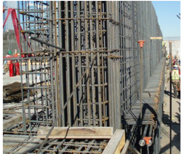
Fig. 2.6.39: Reinforcement and formwork placement for a deep transfer girder. The wide reinforcing cage below was designed as the reinforcing cage for a beam that will support the transfer girder and its formwork during placement, thus avoiding the need for shoring to support the full weight of the deep girder. (Image courtesy of Ceco Concrete Construction.)
