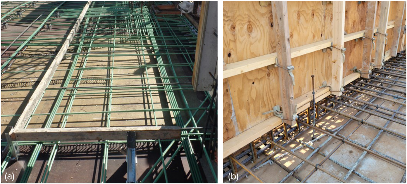
Fig. 2.6.31: Examples of problematic slab transitions: (a) the forms at this transition are not braced, increasing the risk of displacement during the concrete placement; and (b) this large transition will create high uplift pressures in the lower concrete surface, making it difficult to achieve the required surface finish. (Images courtesy of Ceco Concrete Construction.)
