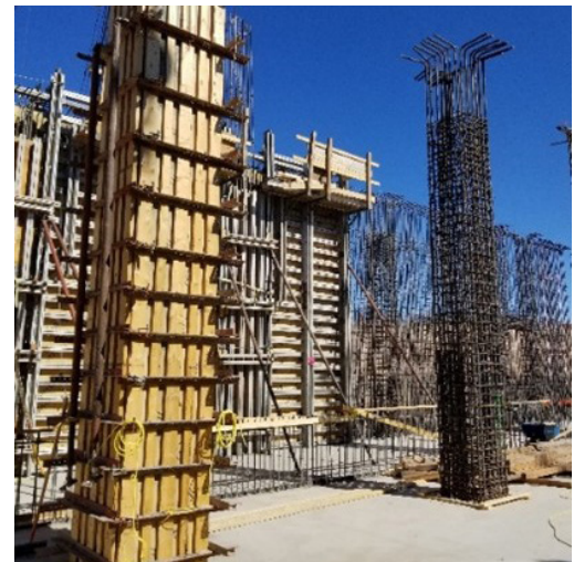
Fig. 2.6.2: When possible, use the same column size and geometry over the full area of the building and maintain column sizes over at least 10 floors. (Image courtesy of Ceco Concrete Construction.)
