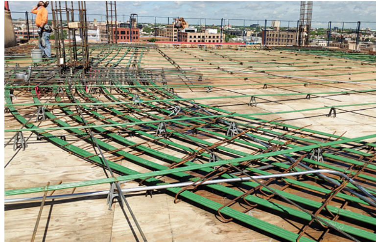
Fig. 2.7.51: Tendon sweeps should be anchored with hairpins if tendons are near slab openings and sleeves. (Diagram and image courtesy of Amsysco.)
