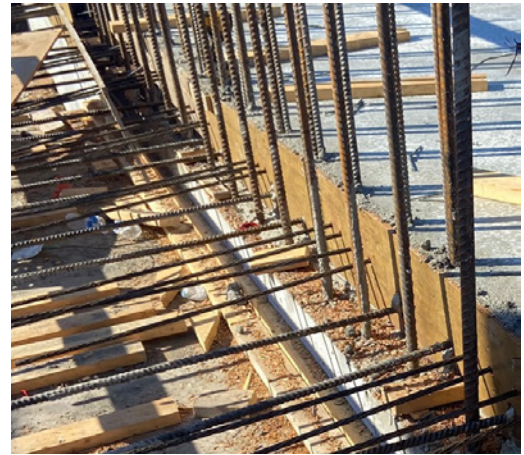
Fig. 2.6.11: Details requiring formwork surfaces to be penetrated by PT strands and reinforcing bars will mandate labor-intensive removal of forms and consume formwork materials. While the shown penetrations are not on a gang form, they may have prevented the use of such a productivity enhancing form system. (Image courtesy of Ceco Concrete Construction.)
