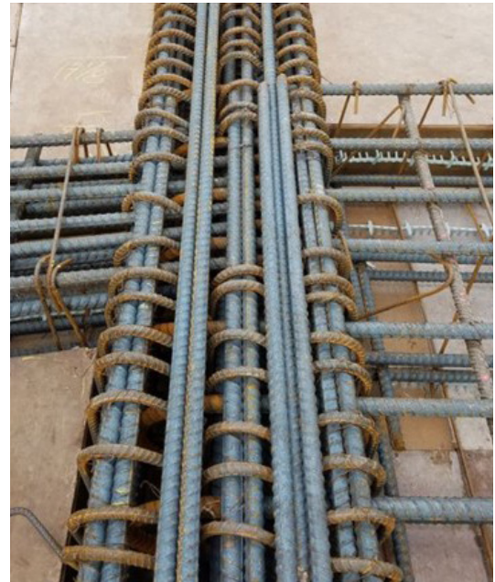
Fig. 2.2.1: Designers must be aware of the need to place and consolidated concrete. (Image courtesy of Ceco Concrete Construction.)
