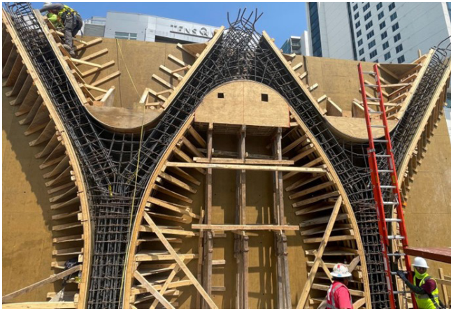
Fig. 2.6.16: An extreme example of an unusual and expensive column shape. Such features should be limited to structures in which such architectural statements are desired. (Image courtesy of Ceco Concrete Construction.)
