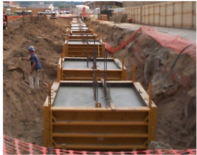
Fig. 2.6.24: While designing footings to have matching depth and alignment aids in constructability, even greater constructability may be achieved by replacing closely spaced footings with a continuous footing. (Image courtesy of Ceco Concrete Construction.)
