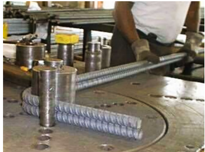
Fig. 2.7.9: A worker uses a bar bender to fabricate standard 90-degree hooks on two No. 9 bars. (Image courtesy of CRSI.)
