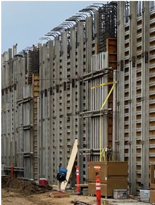
Fig. 2.6.9: Example of gang wall formwork with non-drafted pilasters. (Image courtesy of Hensel Phelps.)
