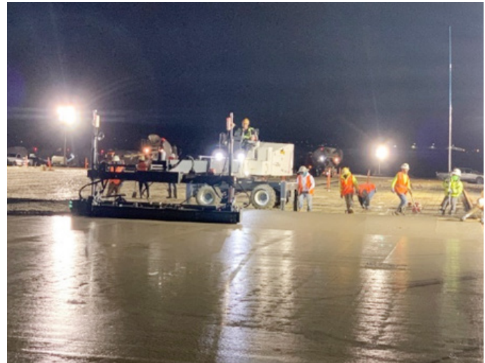
Fig. 2.7.5: A laser screed allows contractors to precisely strike off the concrete during slab-on-ground construction. (Image courtesy of Somero.)
