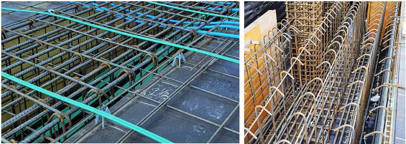
Fig. 2.7.24: Wide beams with multi-leg stirrups, open to the top. The beam cage can be closed using a separate top cap. (Image courtesy of Conco.)
