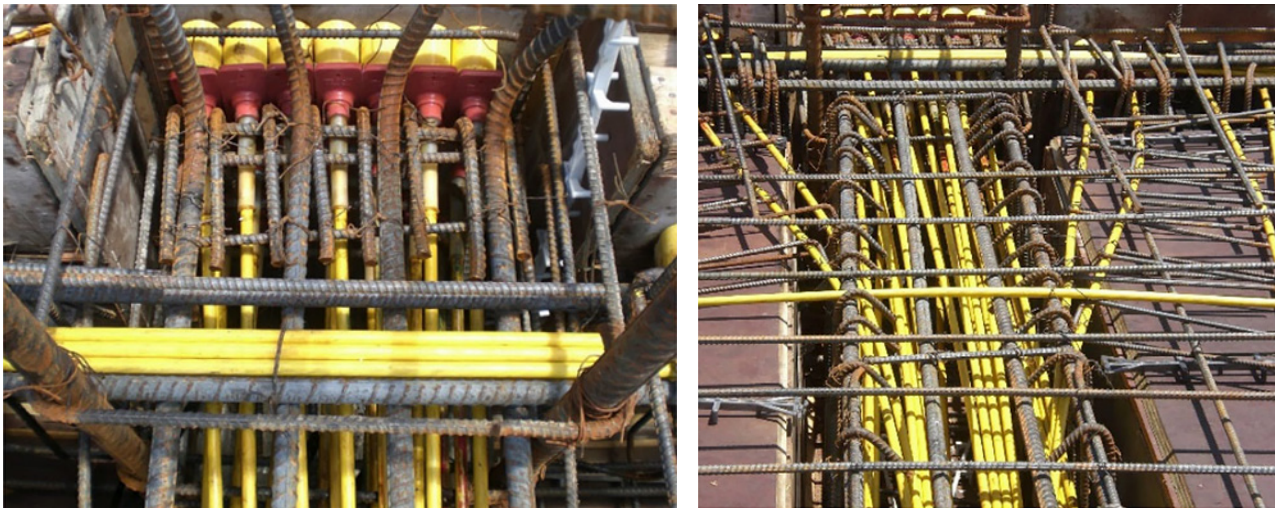
Fig. 2.7.45: Congestion in anchorage zones may prevent concrete consolidation. (Images courtesy of PTI.) Stacked and abutted PT tendon anchors indicate the beam width is insufficient for constructability. The most preferable solution would be widening the beam. Additional solutions could include flaring more cables, eliminating embedded items and MEP items in the congested zone, using headed bars or stud rails in lieu of hooked bars, or even using a multi-strand bonded PT system in the beam.
