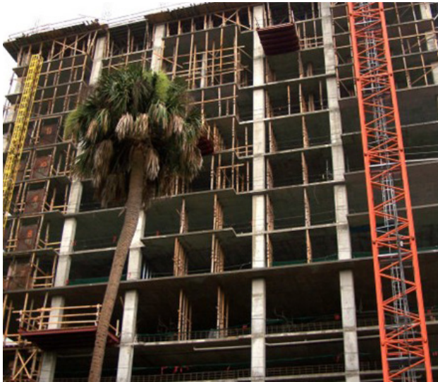
Fig 2.6.38: This project included an upper-level floor with a large dead load. Seven levels of reshores were needed to support the placed concrete. The reshores delayed finish trades in the affected levels and extended the overall construction schedule until sufficient concrete strength was attained on the freshly placed level to allow removal of shoring. (Image courtesy of Mary Bordner Tanck.)
