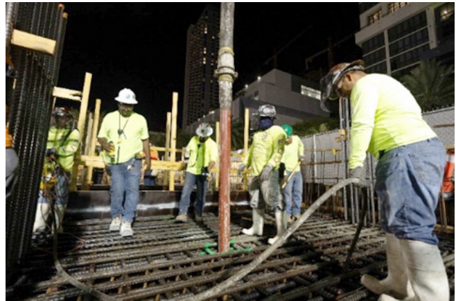
Fig. 2.7.2: Early communication between the contractor and designer resulted in the development of preplanned openings in the reinforcing mat for insertion of the concrete pump hose. (Image courtesy of Ceko Concrete Construction.)
